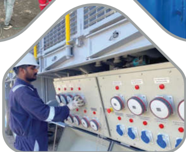
CUSTOMISED PANEL FOR RIG APPLICATION
